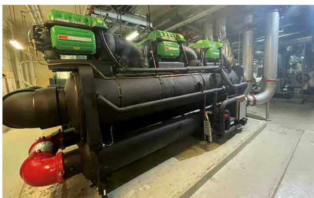
The upgrading of the air-conditioning chillers at 508 Chai Chee Lane was completed in September 2023
