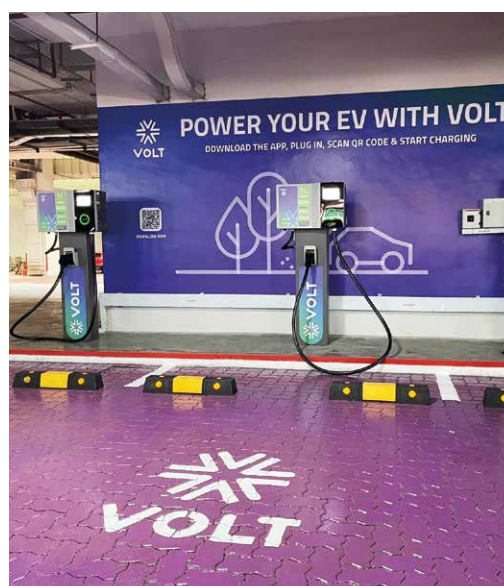
Electric vehicle charging stations at New Tech Park
