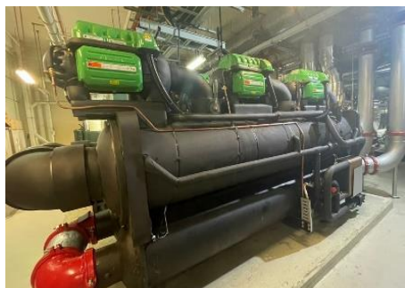
Upgraded air-conditioning chillers at 508 Chai Chee Lane
