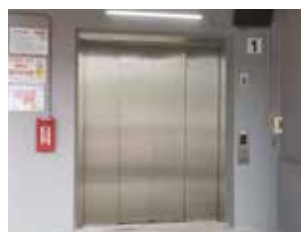
The replacement of two cargo lifts at 10 Changi South Street 2 was completed in 4Q 2021
